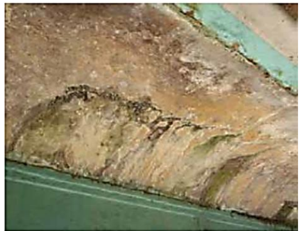
evidence of water ingress to jack arches
