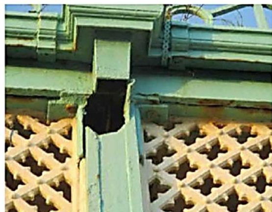
collapsed rainwater downpipe
