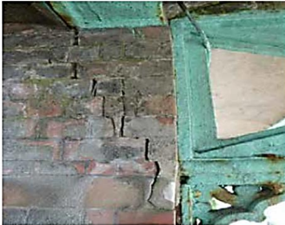
fracture in brick support structure
