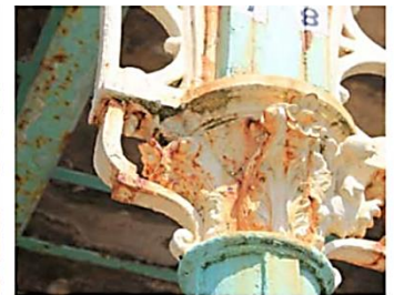
corrosion through paintwork
