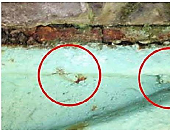
bolted connections failed
