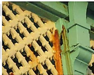
corrosion through paintwork
