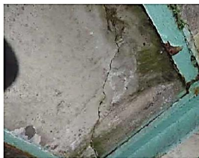
cracks in concrete jack arch
