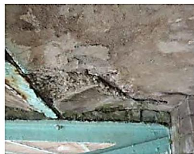
spalling, decaying jack arch
