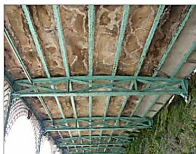
extensive weathering, cracking and spalling
