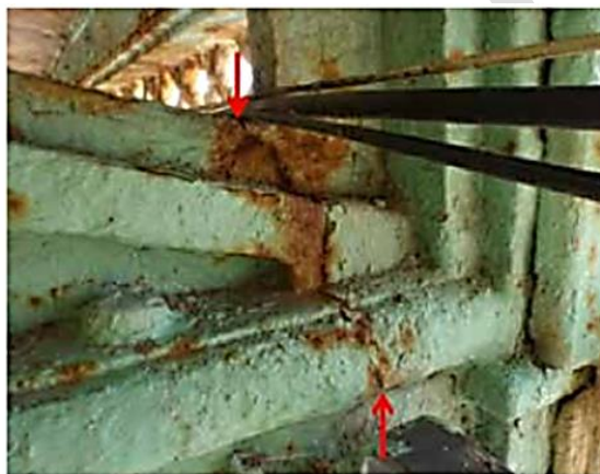
lattice beam failure
